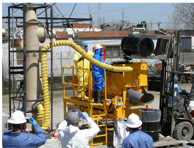
Fig. 1. Picture of the pugmill equipment used in the pilot program during pilot program execution.
